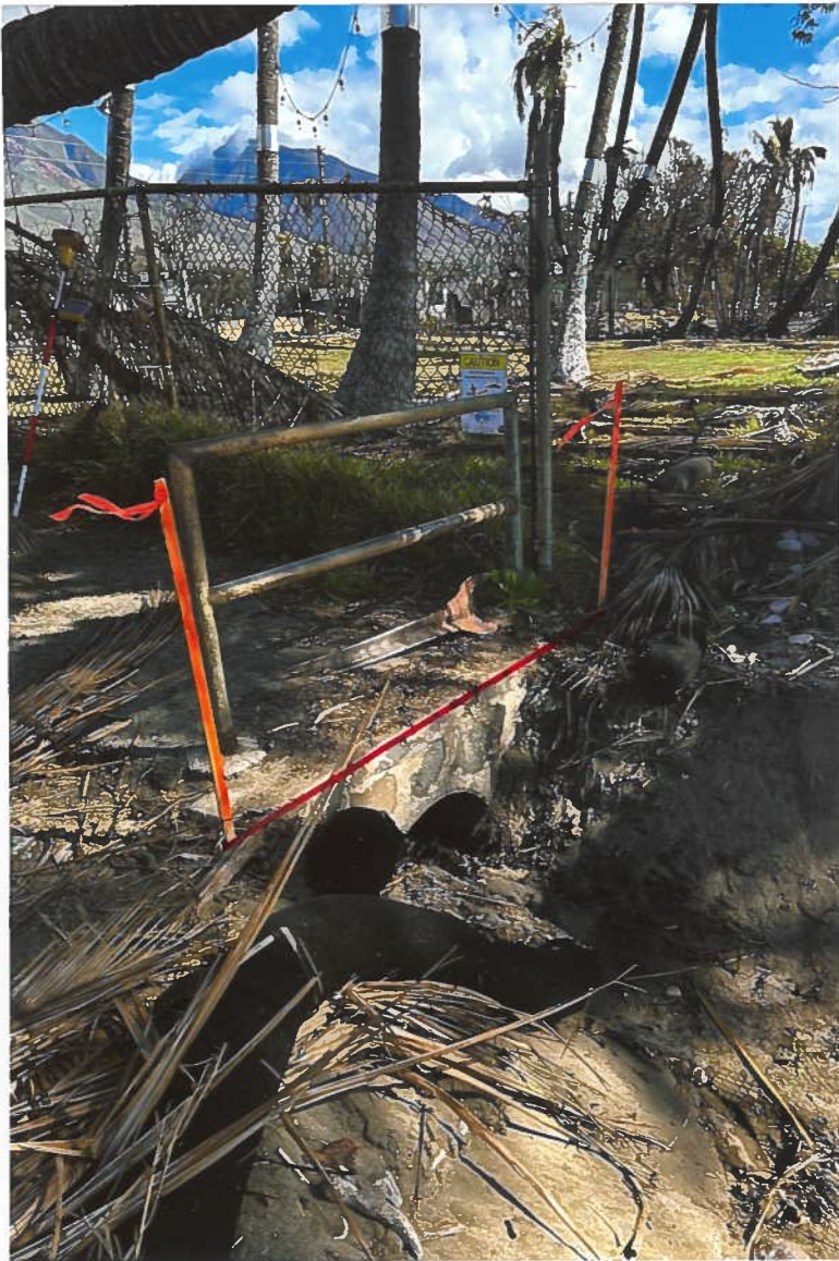
PICTURE # 1: SHORELINE TMK: (2) 4-6-002:002 AT 2:00 PM ON FEB. 29, 2024.
