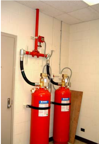
FM-200 Fire Suppression Canisters Installed in SRC
