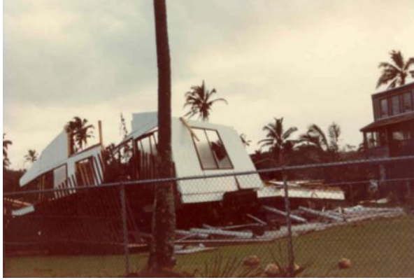
Example of severe hurricane damage to a home: loss of roof sheathing and roof framing structure, windows breached by windborne debris, and failure of wood foundation posts and beams.
